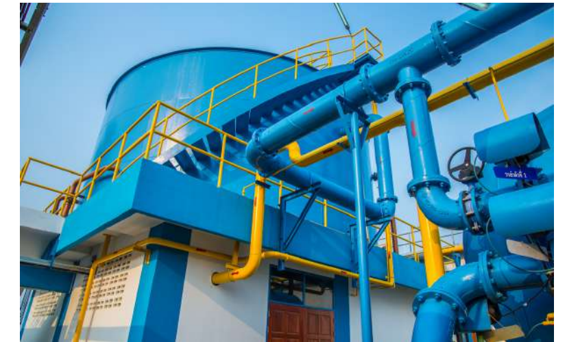
WATER PLANT & PIPELINES
