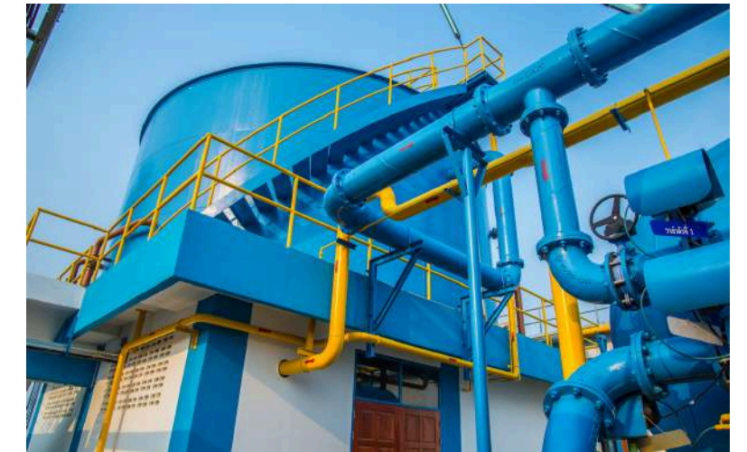
WATER PLANT & PIPELINES
